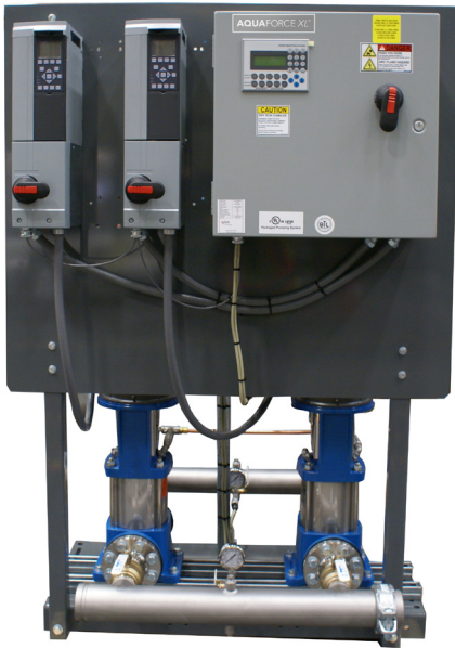
AquaForce (2-4 pumps and max 75 HP)
